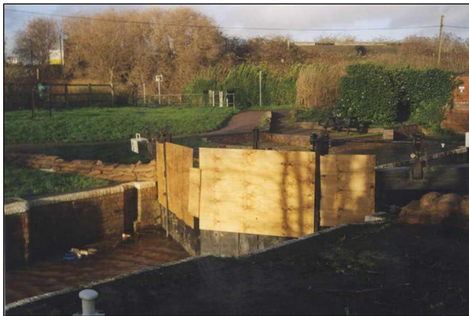
Figure 4 – Emergency works to Firepool Canal lock gates to prevent Tone water entering the canal in 2000. (Environment Agency).
